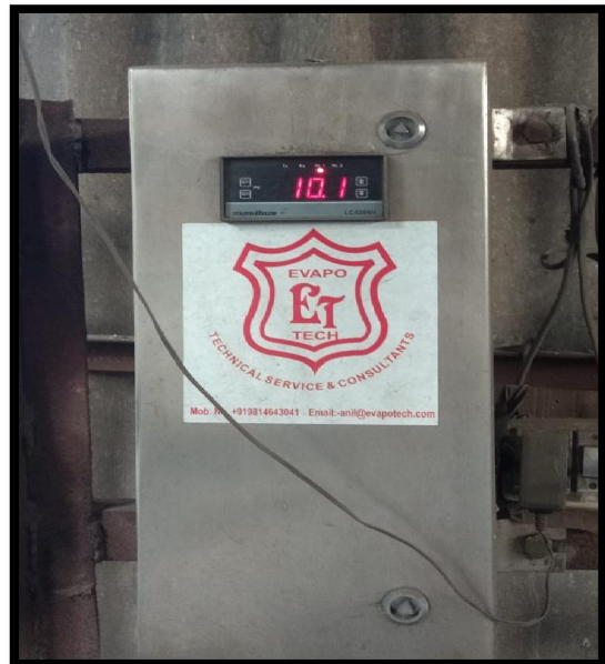
Photographs showing OCEMS installed
