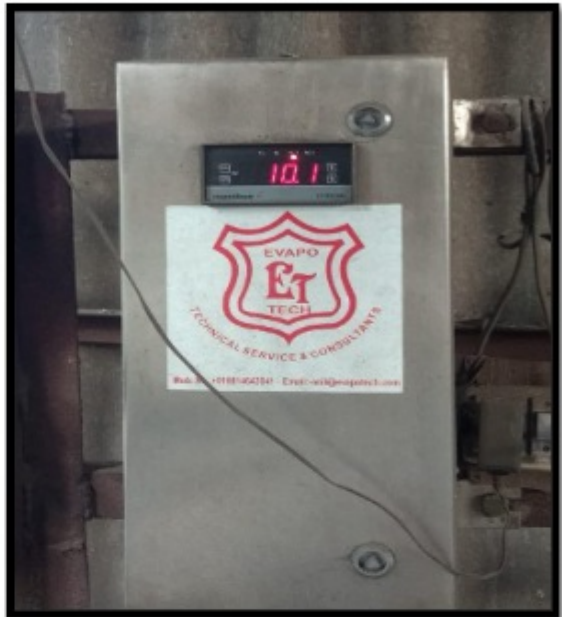
Photographs showing OCEMS installed
